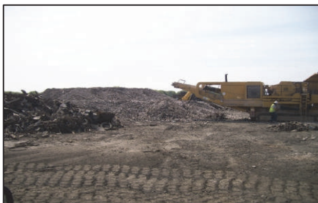
Figure 11b Crushing operations - over 12,000t processed and re-used within the new Development Platform
