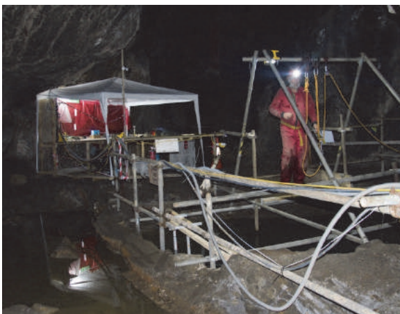
Figure 10: The launch platform, and the adjacent work station, at the pumping shaft, photographed as their installation was being completed
