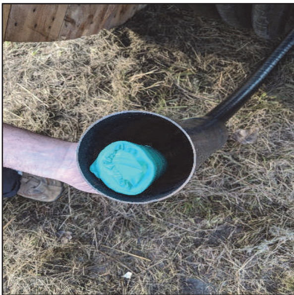
Figure 14a 400V DC cable shown within the 110mm Ø duct
