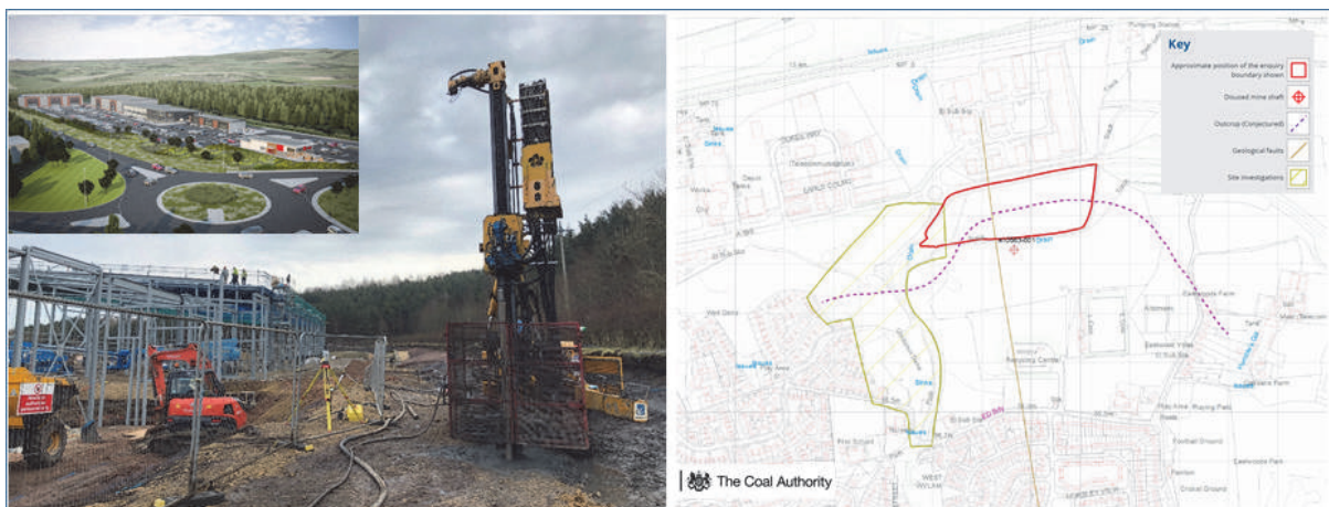
Figure 3: Tyneview Retail Park, Prudhoe. Grouting works and superstructure construction underway in March 2020 site inspection photo (left) and developers completed scheme visualisation (inset top left). Coal Authority consultants mining report plan extract, September 2018 (right).
