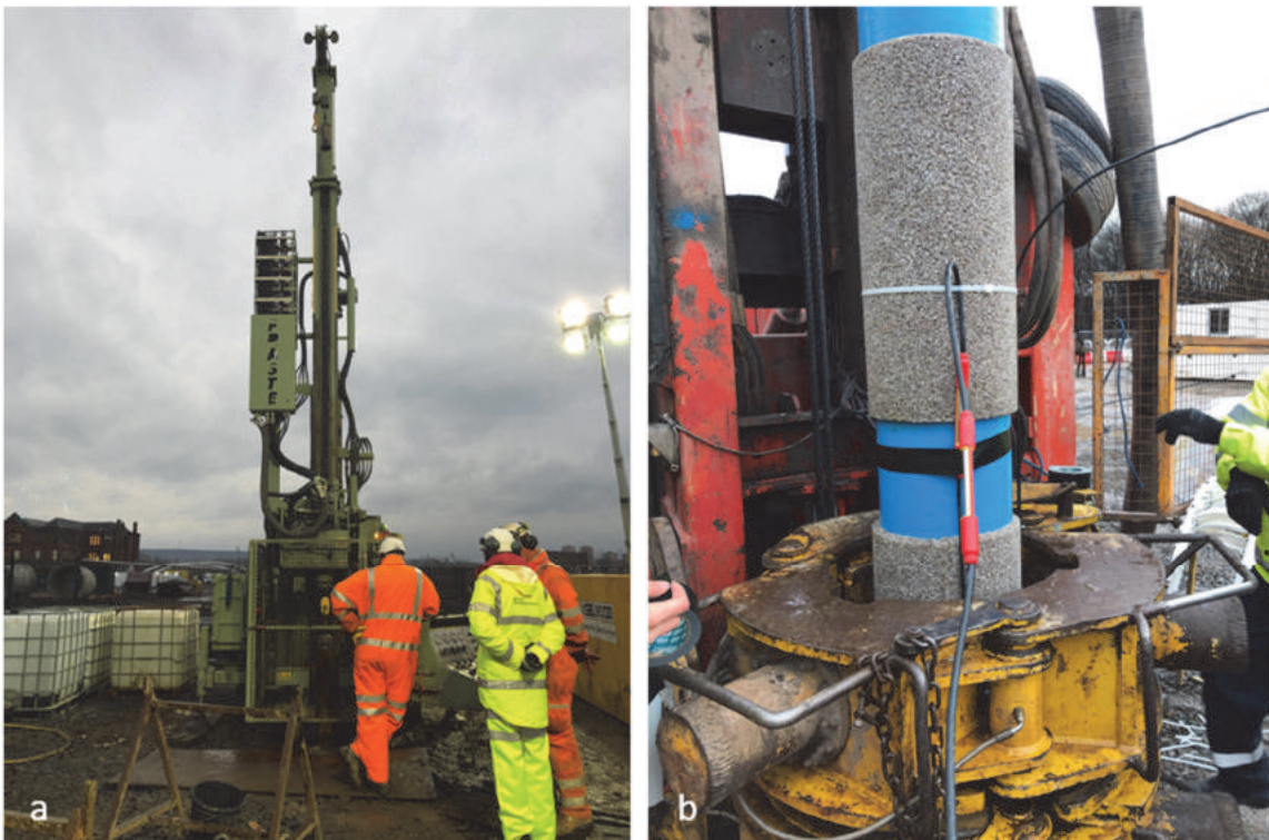
Figure 2: (a) Drilling of the cored borehole GGC01 (b) Installation of uPVC casing screen to mine water borehole GGA08, with pre-glued gravel pack and electrical resistivity sensor cable being attached (red sensors). Photos ©BGS/UKRI 2020.
